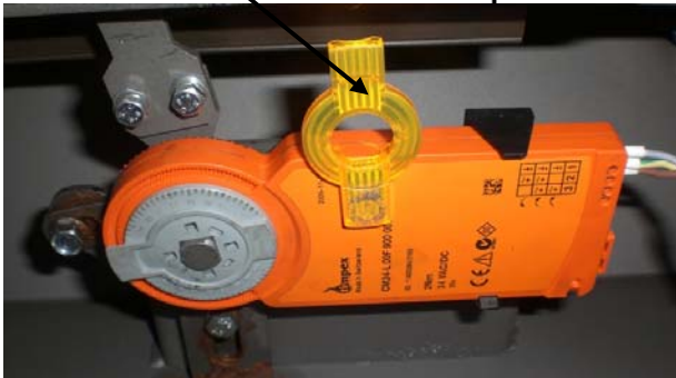
Instructions mode during a power failure
